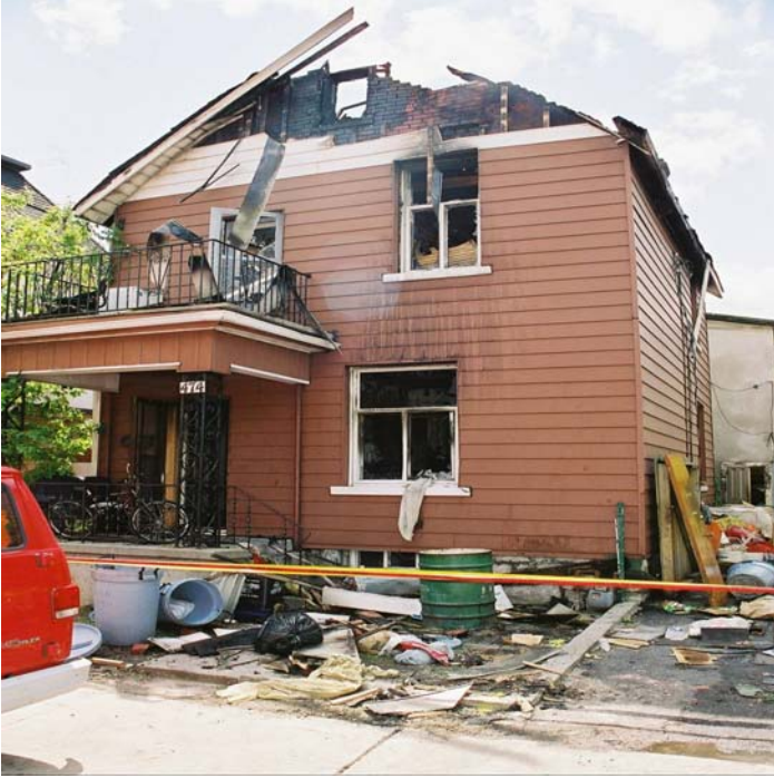
Photo Fire; Furnace fan overheated
