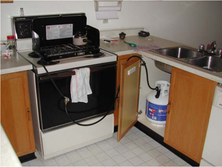
Photo Propane tank ;Potential for explosion
