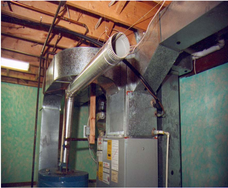
Photo Furnace Alteration; introduces carbon dioxide and Carbon monoxide.
